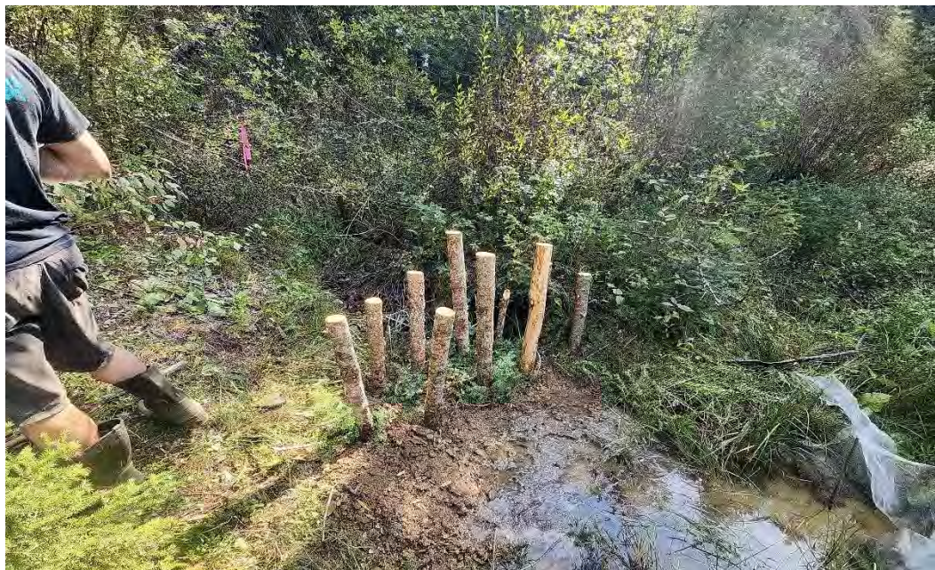
Figure 49. Crews monitor the BDA's performance as water pools behind it, ensuring proper function before increasing its height or installing additional structures in Northbound wetland. September 2025.
