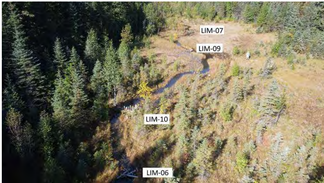
Figure 64: Post-construction drone image in Limbo showing PAL LIM-06, BDA LIM-10, PAL LIM-09, and BDA LIM-07, and associated flooding.
