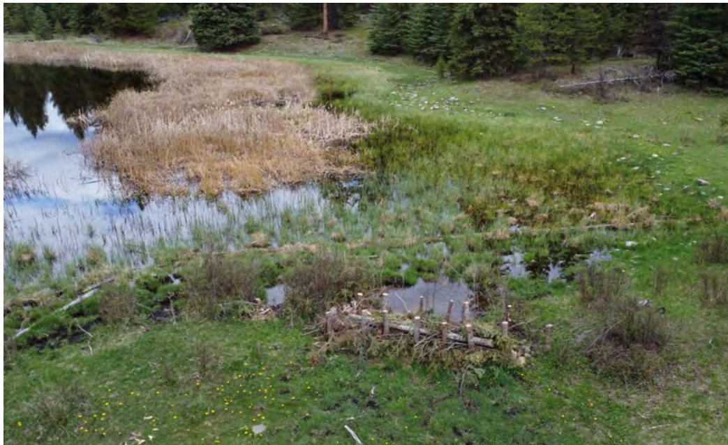
Figure 24. Downstream BDA was constructed at Beaver Channels in September 2024, showing water held behind the dam in May 2025. This area directly behind the BDA was not flooded in May 2024.
