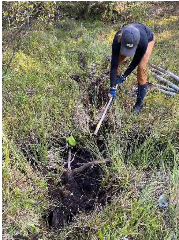
Figure 39. A staff member working during the initial stages of BDA construction at Double Dam restoration site, September 2025.
