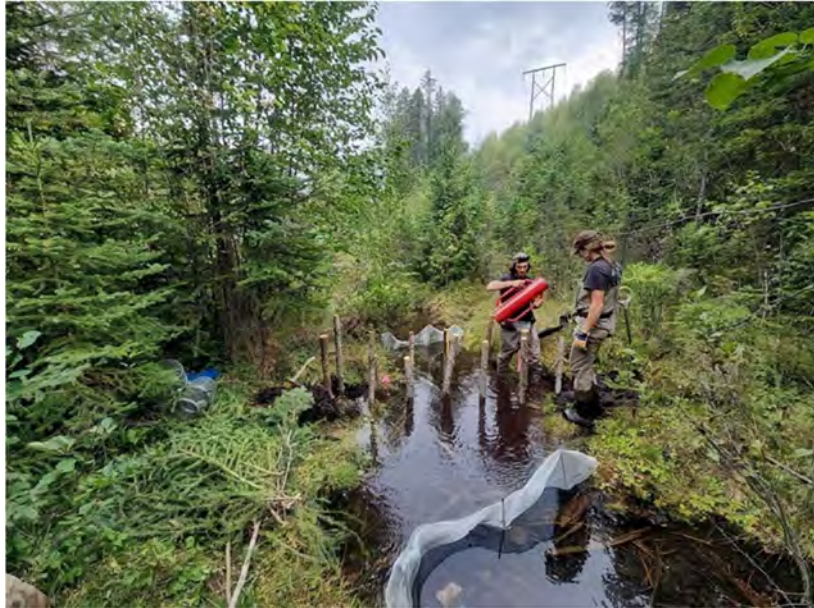
Figure 65: In-stream isolation (fine-mesh window screening secured with rebar posts and rocks) set up around LIM-08 on September 8th, 2025. This image was taken after fish salvage was finished and crews began to install vertical wooden posts in Limbo wetland.
