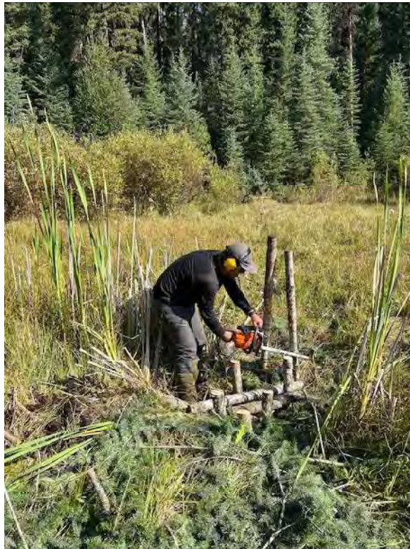
Figure 37. A crew member shortening the posts on one of the Beaver Dam Analogues in September 2025.
