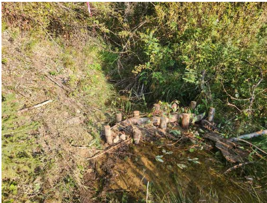
Figure 57. A completed Beaver Dam Analogue that was constructed at Big Dam in September 2025.
