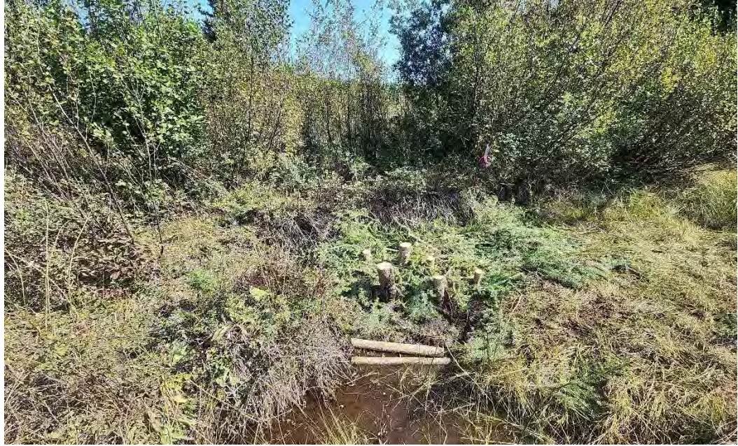
Figure 36. Beaver Dam Analogue was constructed by hand during restoration work at the Double Dam site, September 2025.
