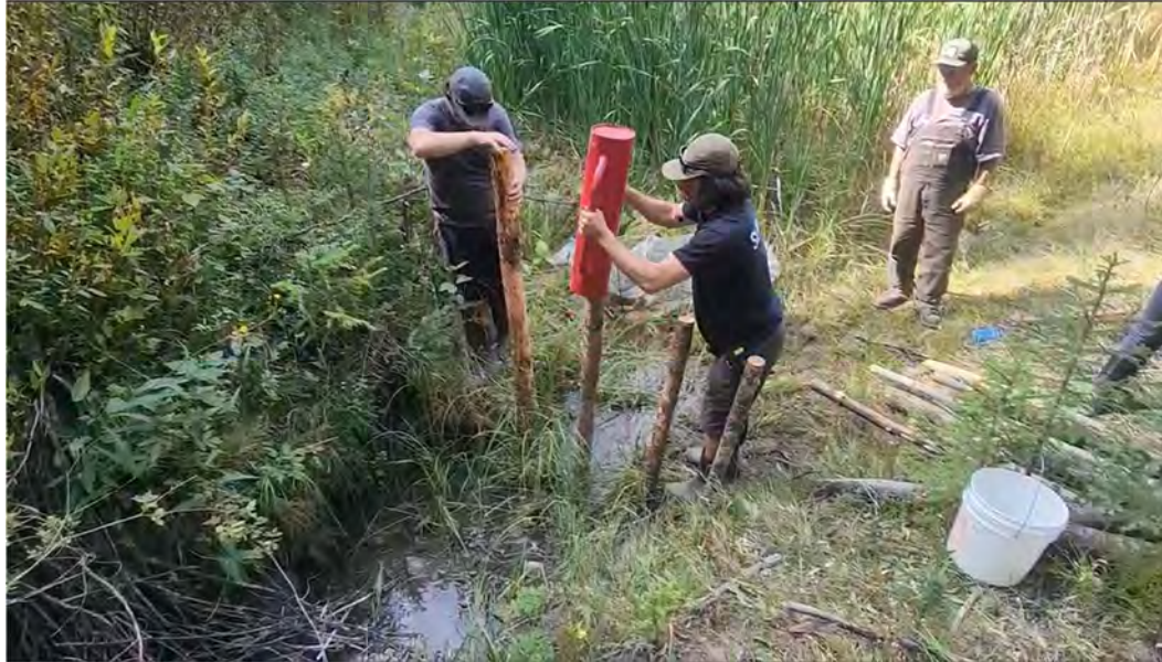
Figure 48. Crew uses a 'post pounder' to secure posts into the ground in Northbound wetland during BDA construction in September 2025.
