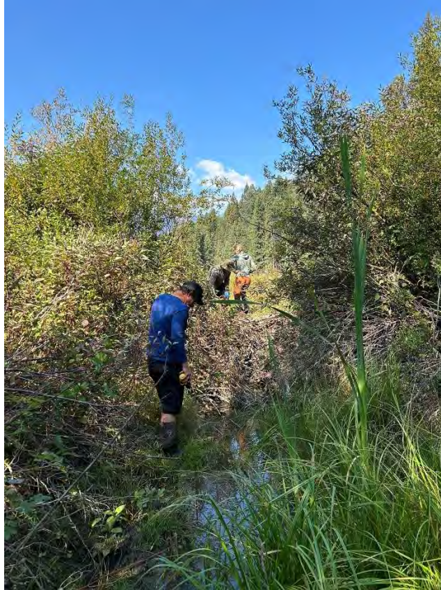
Figure 58. Crews construct a BDA in the background of Big Dam wetland while a team member conducts a visual amphibian survey in the foreground.
