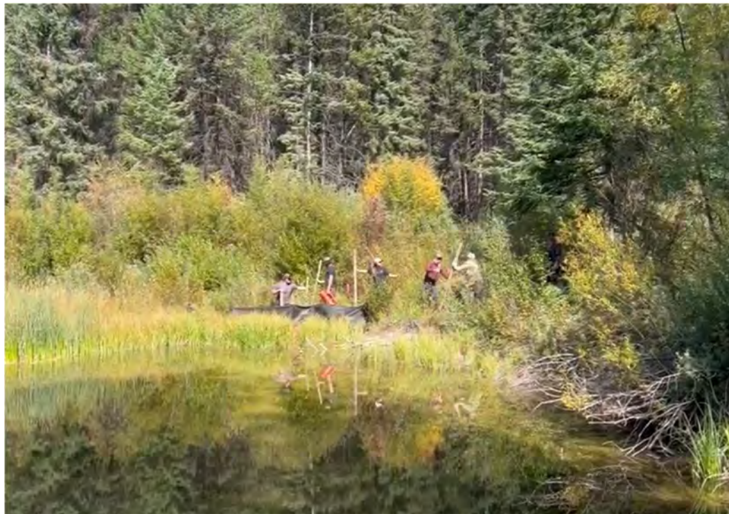
Figure 47. Staff and volunteers constructing a Beaver Dam Analogue at the Northbound wetland restoration site in September 2025. A temporary mesh barrier is visible, functioning both as a turbidity curtain and to isolate the construction area.
