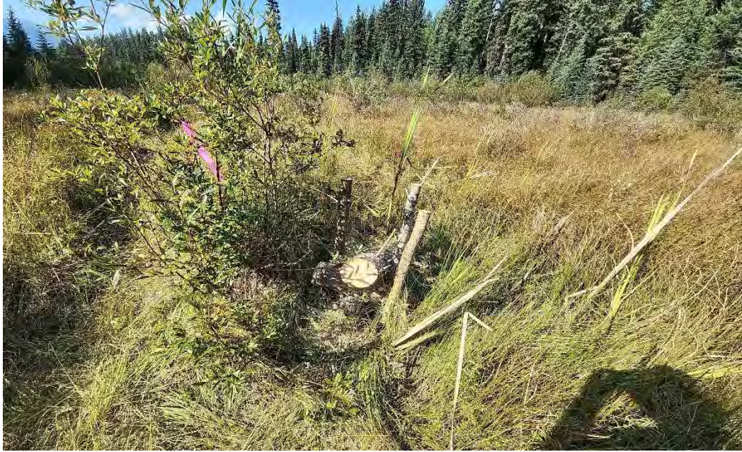
Figure 38. Post Assisted Log Structure was constructed by hand during restoration work at the Double Dam site, September 2025.
