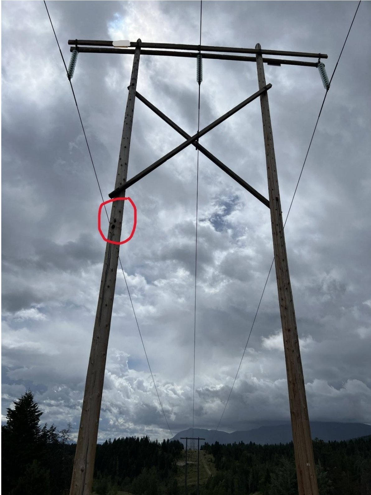
Figure 16. Active nesting cavity in Hydro pole which is being removed in 2026 and replaced with a metal pole.
