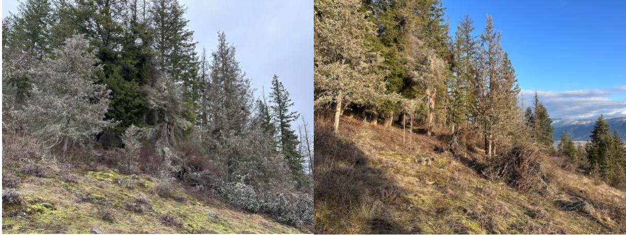
Figure 4 Pre-treatment (left – Jan 14, 2026) and post-treatment (right – Jan 23, 2026) views of thick forested patch brushed and thinned, less than 40m northwest from the CVWMA Office building.
