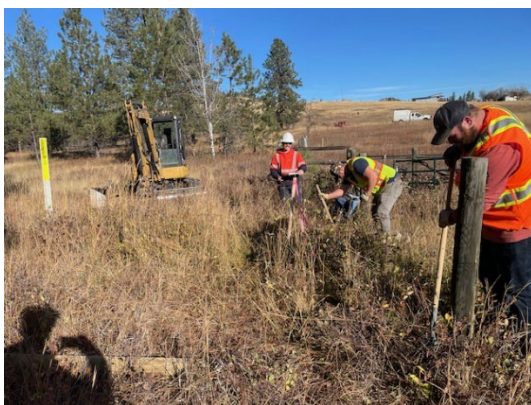
Photo 10: FortisBC overseeing fence post removal and installation in the vicinity of a high-pressure natural gas pipeline, October 2023
