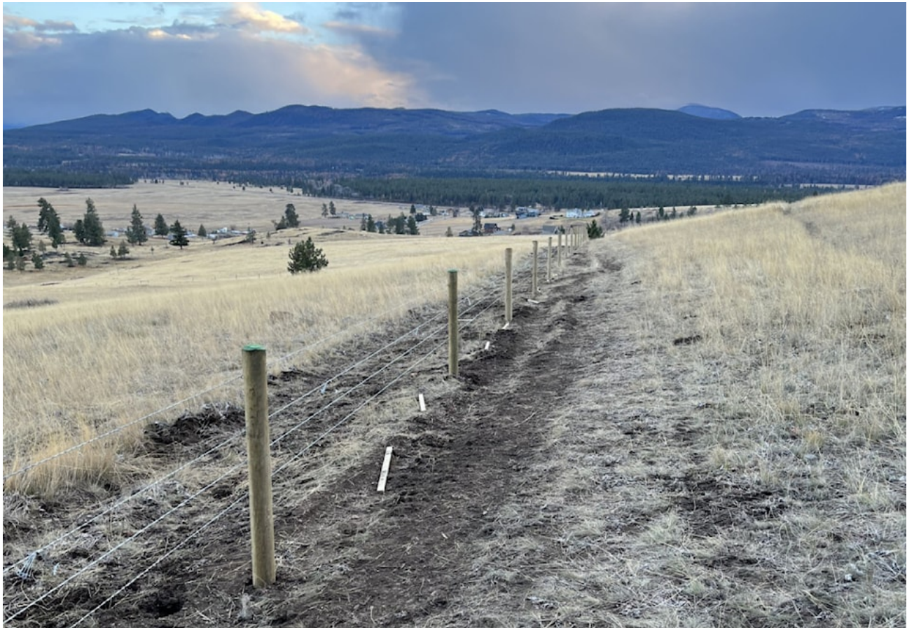
New modified wildlife-friendly fencing (in progress) in Wycliffe Conservation Complex. Chris Bosman/Submitted.
