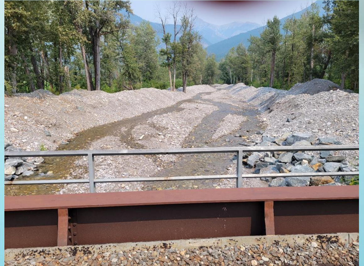
Fraling Creek Reach 1 illustrating the high diversity and high-density electrofishing site. Note the Canadian Pacific Railway Crossing and unstable creek channel associated with substrate removal to protect this infrastructure.
