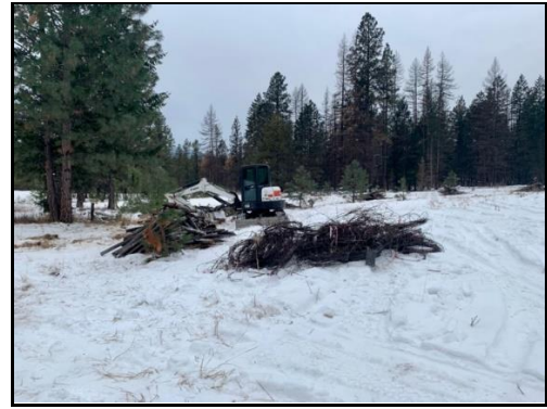
Photo 20: Derelict fence ready for pickup and disposal
